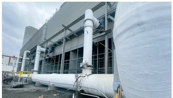
Cooling tower with ruptured beetle pipe.
